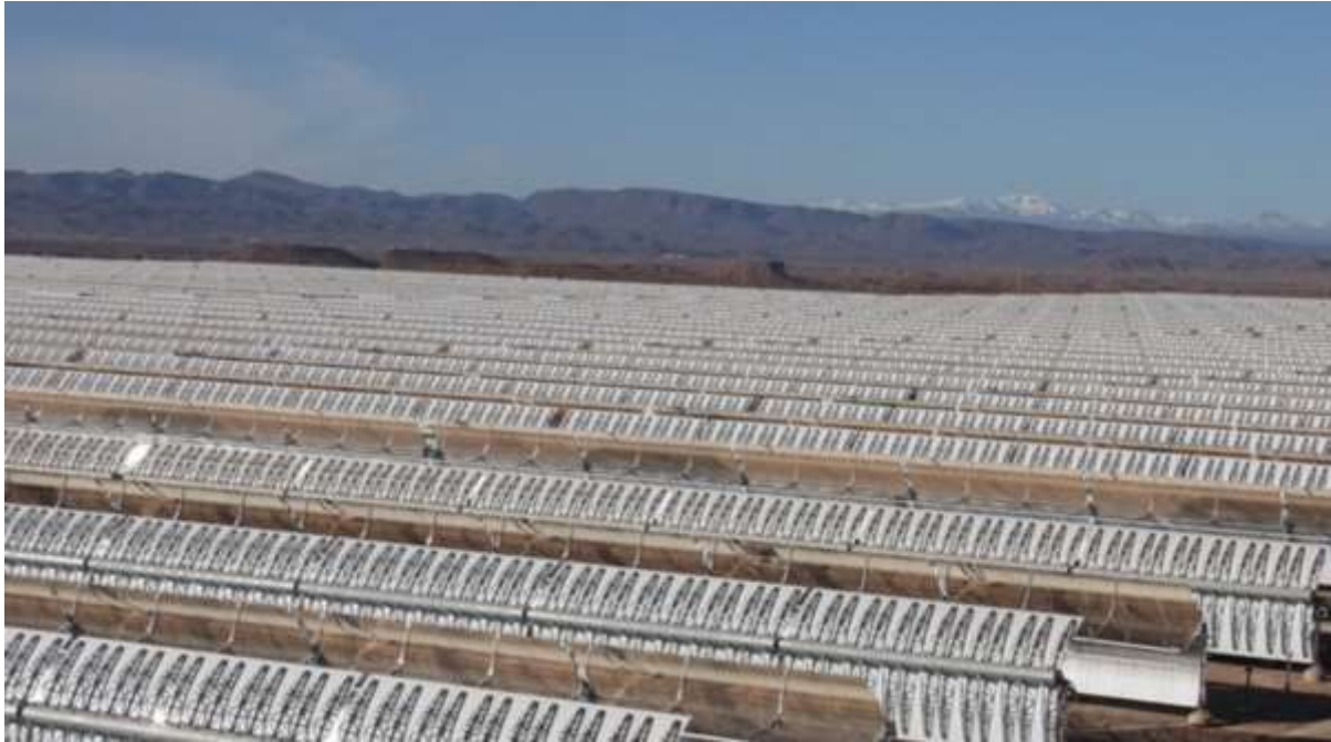
Figure 2 World's Largest Solar Power Generator in Morocco
